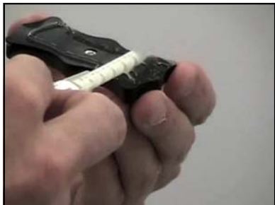
Working quickly, run a bead of Quick Adhesive around the edge of the liner attachment. Smear the bead into a thin layer on the attachment.
